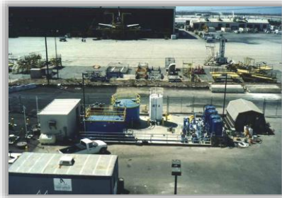
Groundwater Remediation System
